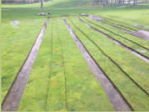
Sod strips removed from first fairway landing area. Ready to be trenched.
